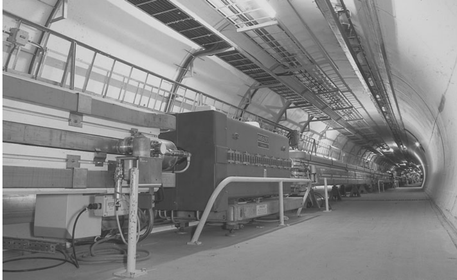
13. A view inside the 27-km (17-mile) circular tunnel of CERN's Large Electron Positron (LEP) collider, which ran from 1989 to 2000. The electrons and positrons travelled in opposite directions in the beam pipe through hundreds of brown and white bending magnets (dipoles) and blue focusing magnets (quadrupoles). Originally LEP accelerated the beams to a total collision energy of around 90 GeV, but by the time of its final shutdown in October 2000 it reached more than 200 GeV.
